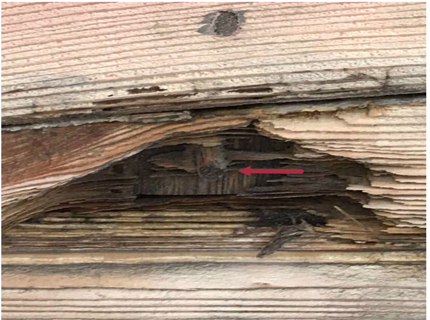
FIG 3. THE DAMAGED PINE WOOD (SOFTWOOD PARTS EATEN AWAY), BUT UNDERNEATH, THE UNDAMAGED OAK TENON AND OAK DOWEL CAN BE SEEN (RED ARROW). PHOTO BY B. DREYER
